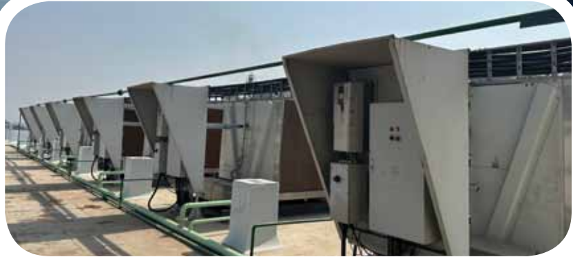
Large scale super adiabatic cooler- Vadodara complex
