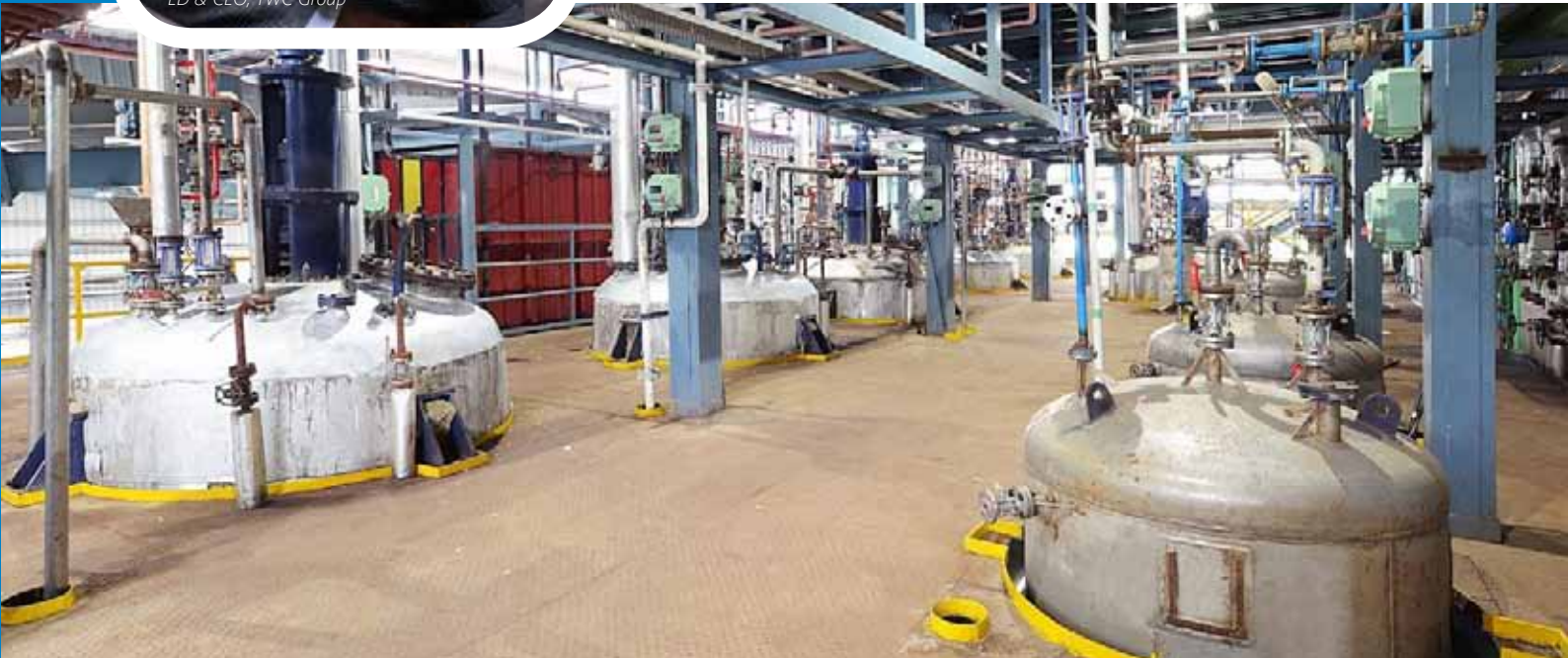
Reactors Train at Vadodara complex
